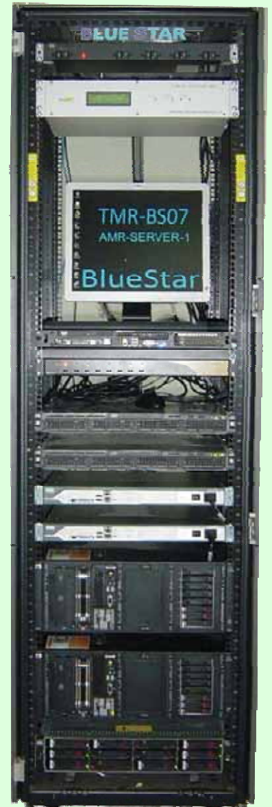
TMR-BS07 System Rack
